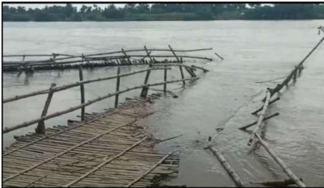
Breakdown of a Bamboo made bridge on mundeswari River beside the Chabbishpur Village
