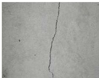
Figure 4. The crack made in the concrete cube with Bacillus Subtilis embedded in it.
