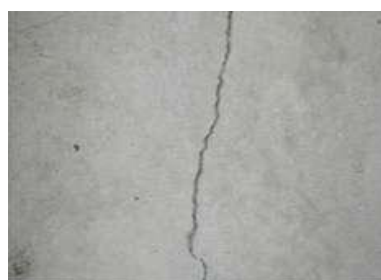
Figure 5. The crack made in the concrete cube with Bacillus Subtilis embedded in it after Self-healing.
