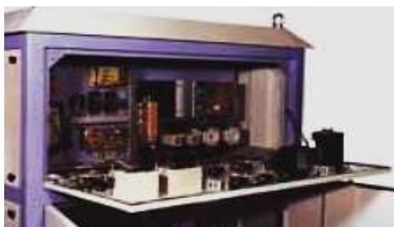
Figure 3. ECM Control Panel.
