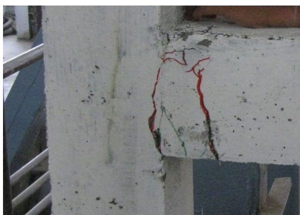
Figure.9 Failure Mode - (PP 50% +Steel 50% ) 2.0 BC Joint
