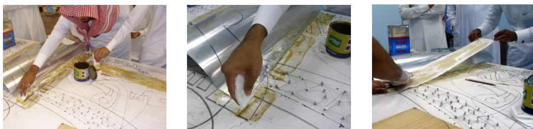
Figure (16) The stage of installing the metal part on the surface of the mural, which represents an element of the buildings of King Faisal University
