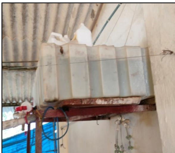
Fig. 6; DRINKING WATER TANK (2.0ppm)
