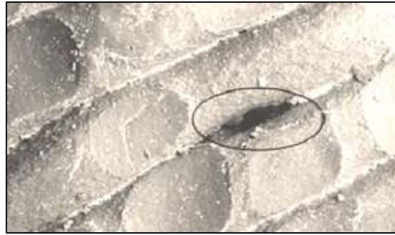
Fig.18.crack between raster (Courtesy Padhi.S.[18])
