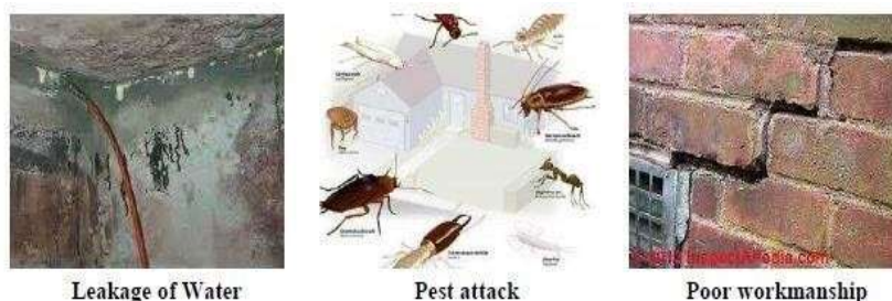
Figure 3. Problems in Expansion Joint
