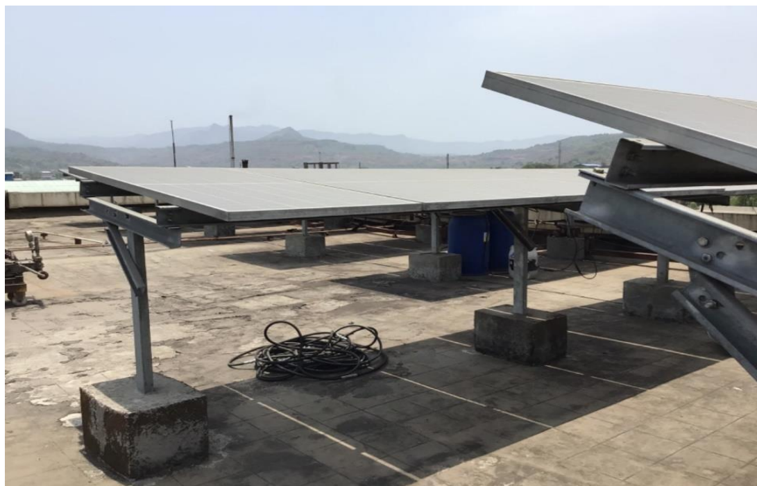
Fig. 6. Uncleaned solar PV panel
