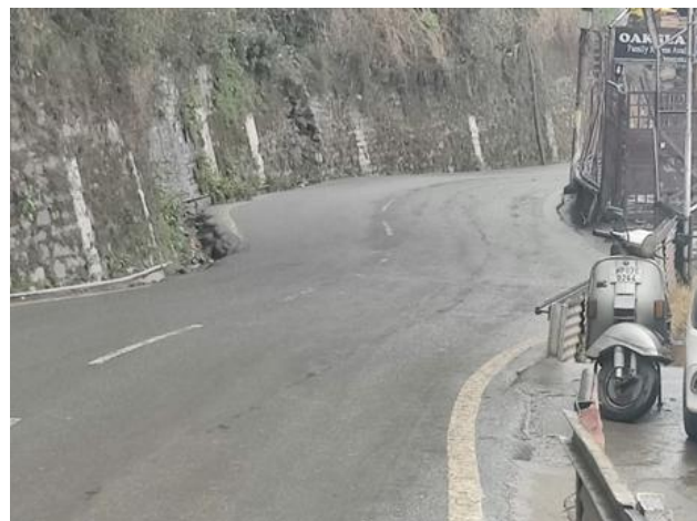
Figure 4 Absence of shoulders
